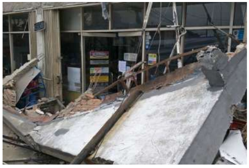
Bangunan Indomart Ambruk, Depok, Senin (6/5/2019)
