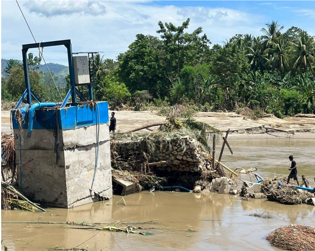
IPA Galung Lombok Rusak, Sulawesi Barat 2022 (Radar Sulbar) https://radarsulbar.fajar.co.id/2022/11/25/instalasi-pengolahan-air-galung-lombok-rusak-ribuan-pelanggan-pdam-majene-tidak-teraliri-air/
